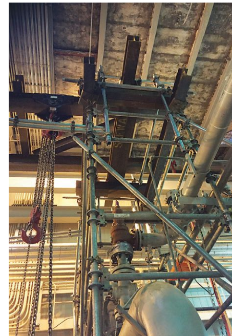
One end of a Safway lifting rig ready and waiting to lift a 32,000-pound valve.
